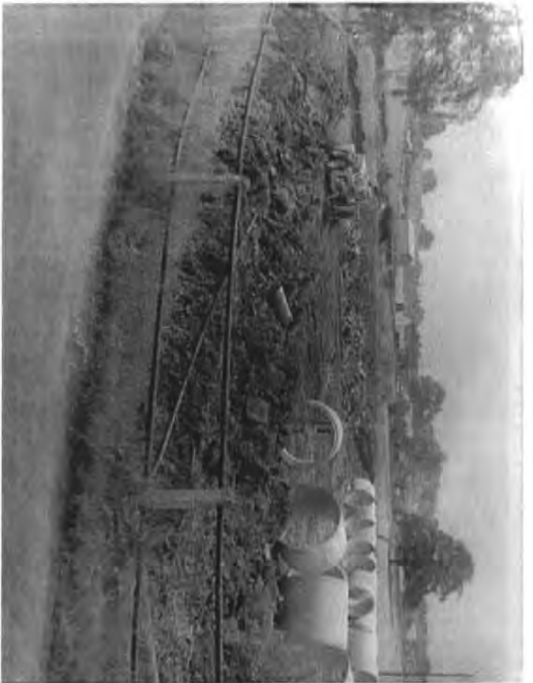
The clearing of the Osier beds and construction of the school playing fields just off Doctor's Lane. All of the civil engineering work was carried out by the Quarry free of charge. The 4ft diameter concrete pipes were sunk into the ground to carry Breecon stream below the surface of the fields. 1960.
