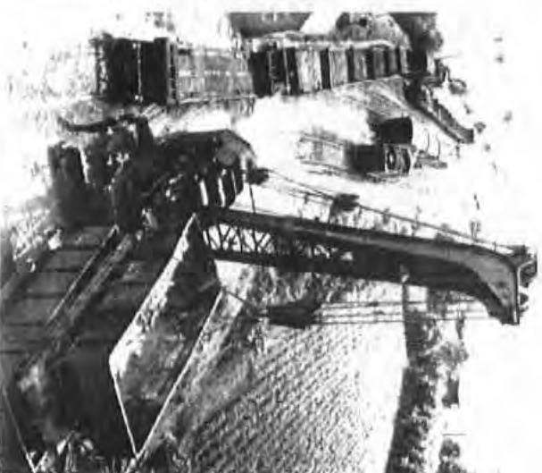
Cleaning away the damaged stone wagons after the incident at Cloud Hill sidings. June 1955
