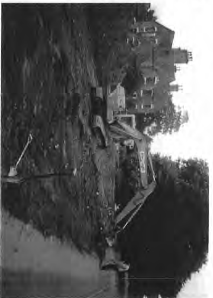
Clearing the site to build 15 new houses, 1999. The new road was appropriately named Henry Dane Way.
